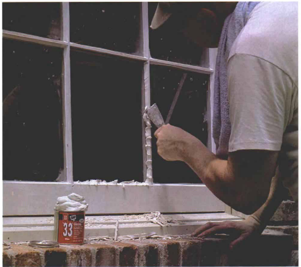
A smooth putty knife removes the excess. Drawing a smooth, clean putty knife along each side of the window at the proper angle presses the compound into place, smooths it out and takes off any excess. The proper angle is determined by the height and depth of the rabbet.
